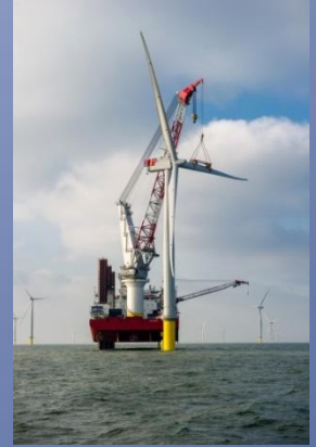
Copyright: London Array Ltd.
